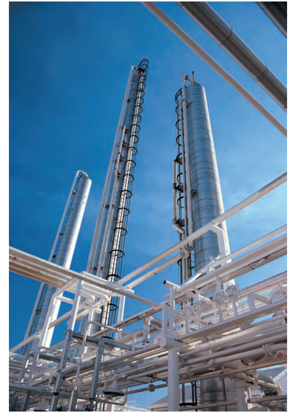
油田管道 Oil Field pipeline
