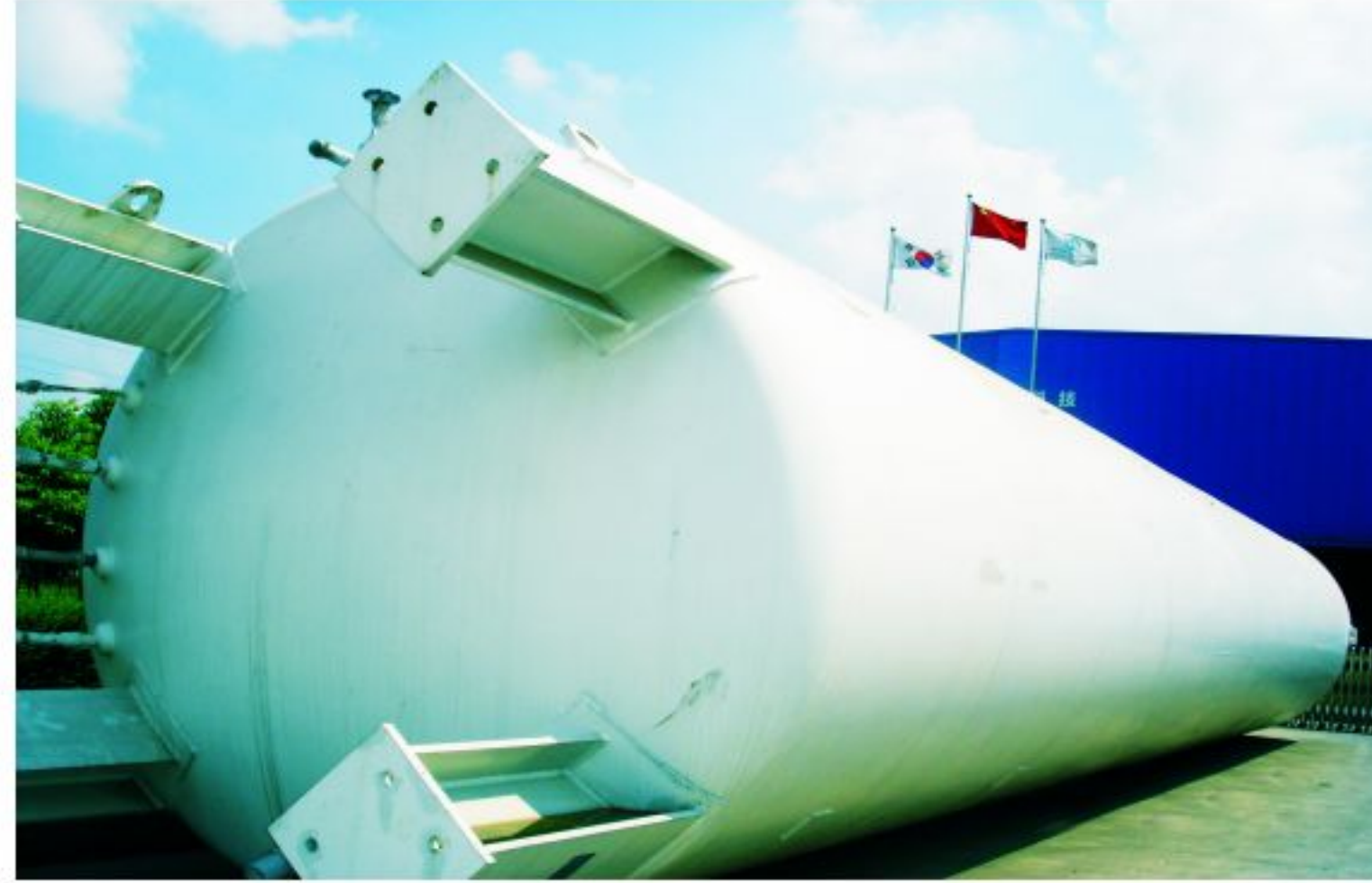
低温液体储罐，内胆材质为16MnDR Low-temperature liquid storage tank, whose inner bladder is made of 16MnDR
