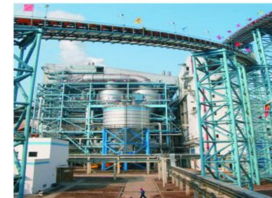
电站锅炉 Power station boiler
