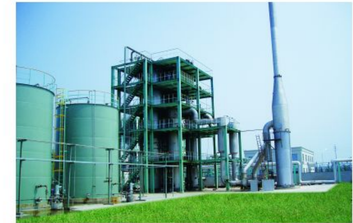
垃圾焚烧厂 Waste calcinations plant
