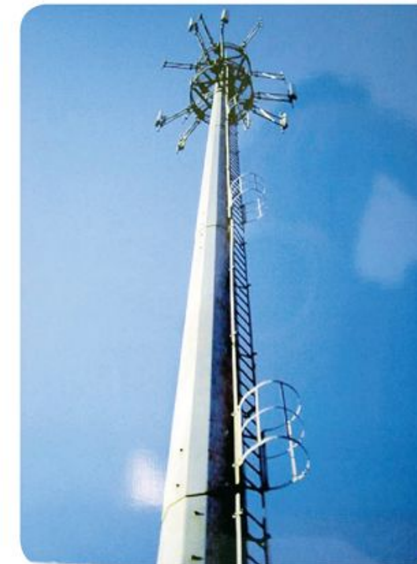
通讯塔 communication tower
