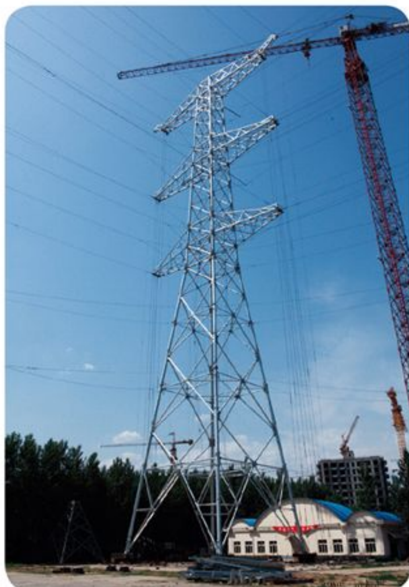
1100KV特高压输电铁塔 1100KV Extreme voltage transmission iron tower
