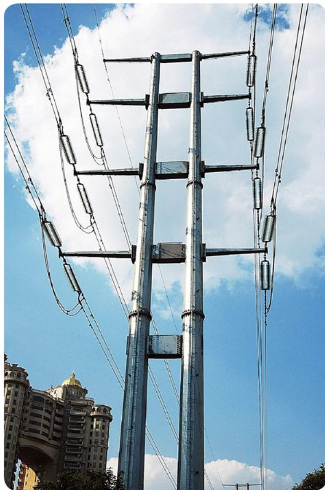
输电杆塔 Transmission pole and tower
