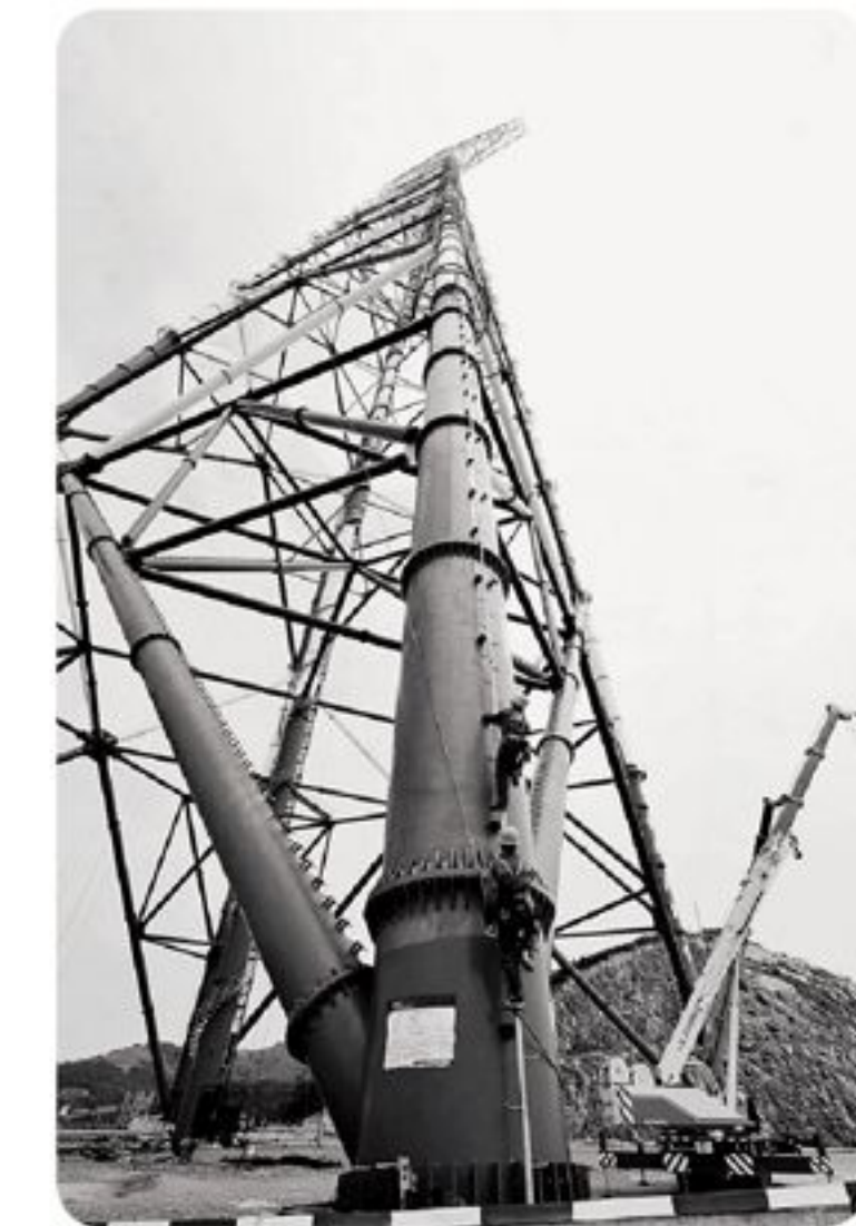
钢管塔 Steel pipe tower
