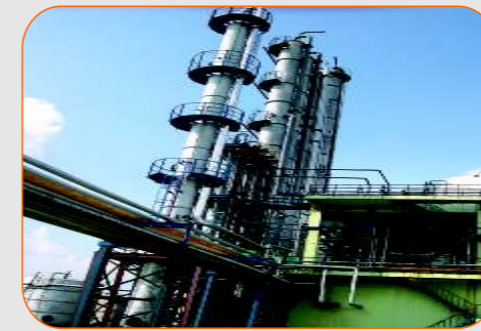
炼油蒸馏装置 Refining and distilling equipment
